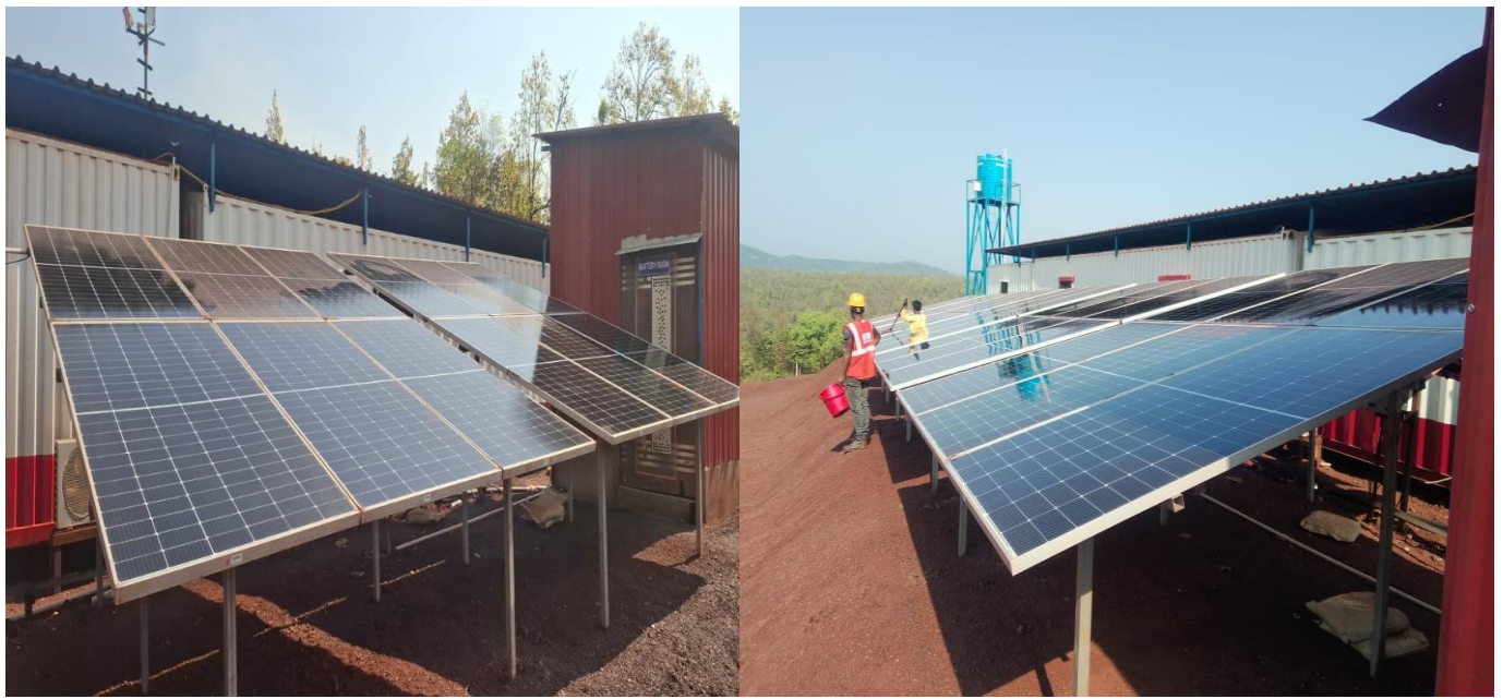
Photo-12 Solar power plant with 30KVA capacity Within the lease area.
